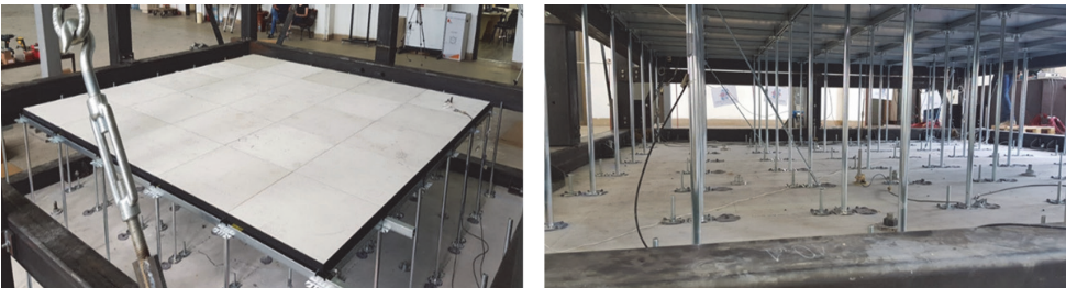
Figure 2. Five by five panel configuration – left. Raised floor structure – right
