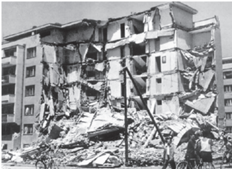
Figure 3. Total collapse of URM building, Skopje 1963
