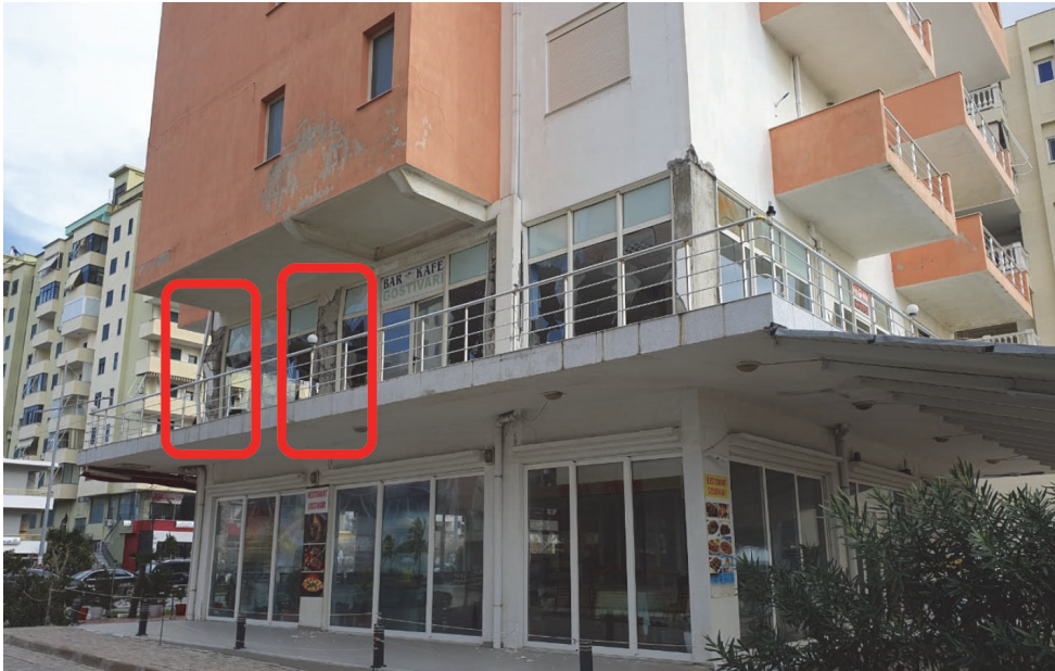
Figure 11. Structural damages by the November 26, 2019 earthquake
