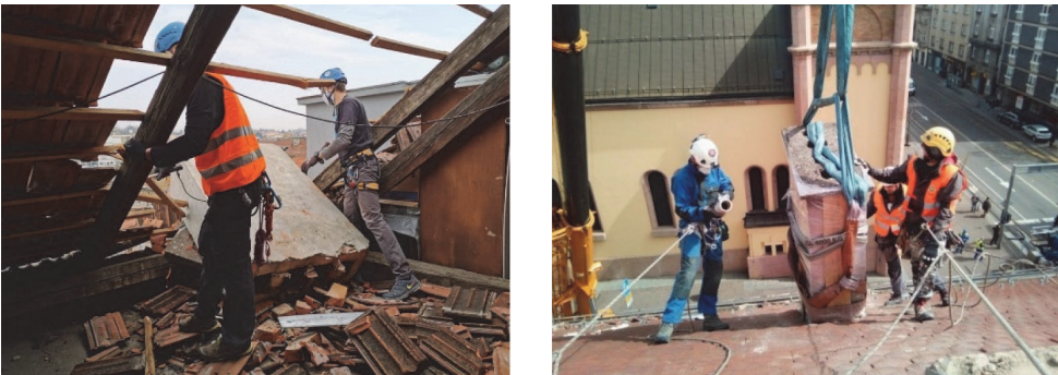
Figure 1. Toppled chimney (left) and the removal of damaged and potentially hazardous chimney (right) after the Zagreb earthquake 2020 [1]
