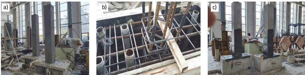
Figure 4. Construction of the models: a) Model M1 and Model M2; b) Construction of the column models for experimental tests; c) Photos taken during application of FRP
