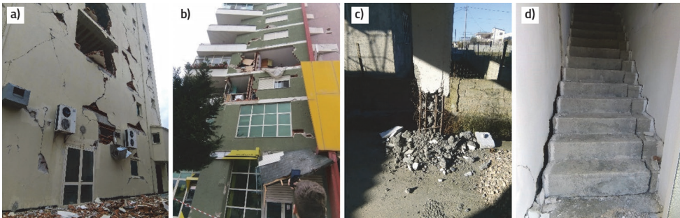
Figure 3. Structures with major non-structural damage (a, b) and Residential structure GF+1 with major structural and non-structural damage, unsafe for habitation (c, d)
