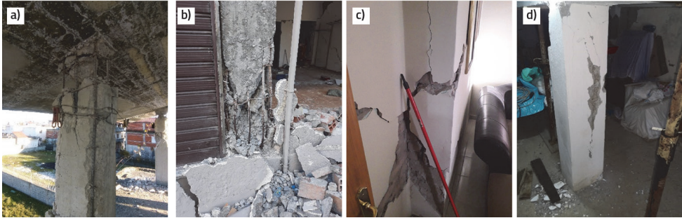
Figure 4. Residential structures: GF+2 (a, b); GF+3 with RC frames at the ground floor and masonry along storeys – visible damages to columns at the ground floor (c, d)
