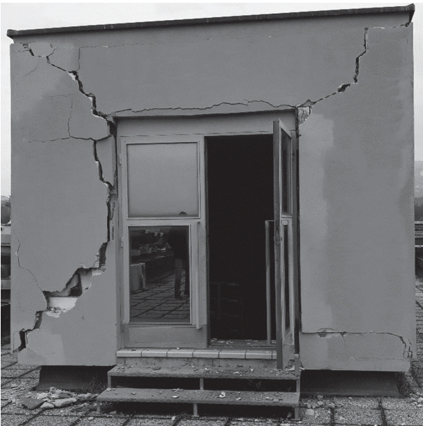
Figure 1. Masonry building damaged in the Zagreb earthquake
