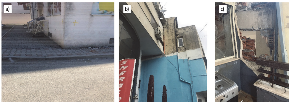
Figure 4. a) Differentiated settlements 1.6% inclination of building. B) Collusion between two buildings different high. C) Bumping effect
