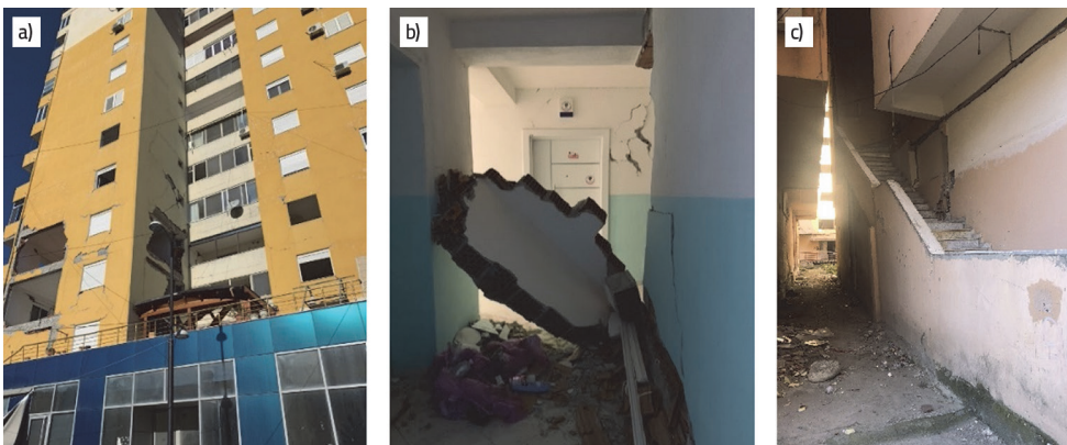
Figure 3. a) Filling walls completely destroyed; b) partitions walls completely destroyed; c) Inclintion and short roblem
