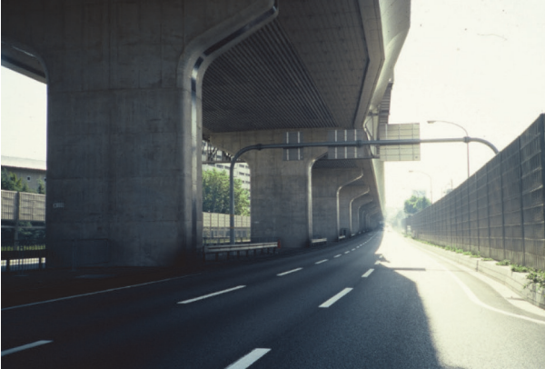
Figure 3. The Fukae section Kobe Route expressway after retrofit implementing measured presented in Fig. 6b (Copyright: M. Čaušević)
