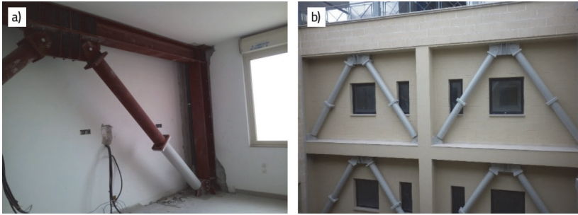
Figure 3. BRAD® as installed in the Altamura Hospital, Italy. Source: [10]
