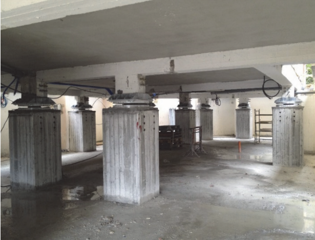
Figure 2. Isolators as installed in an existing building (San Leonardo building in L'Aquila) [11]
