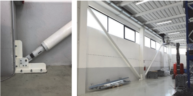
Figure 5. Fluid Viscous Dampers as installed in an industrial building in Italy
