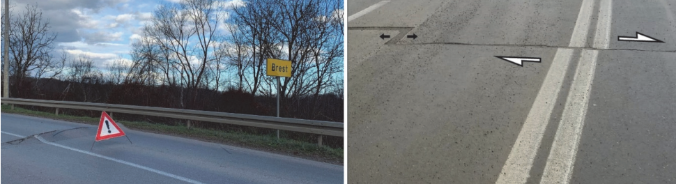
Figure 2. a) Coseismic cracks and small transpressional structure (mole track) along one of the fault lines of the creeping sinistral Petrinja Fault crossing Petrinja-Brest road north of the Brest Bridge over Kupa river (CREDIT: Public media), b) Coseismic dextral ~10 cm displacement (white arrows) and tensional cracks (black arrows) along one of the fault lines of the Pokupsko Fault crossing Petrinja-Glina road west of Župič. (CREDIT: M. Vukovski, HGI)
