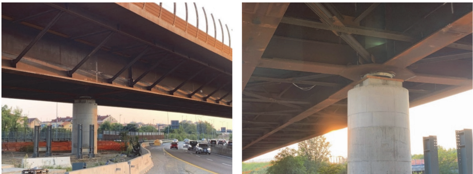
Figure 9. Pendulum isolators as installed in the Rho-Monza Viaduct, Italy (courtesy of Matildi+Partners, Italy)
