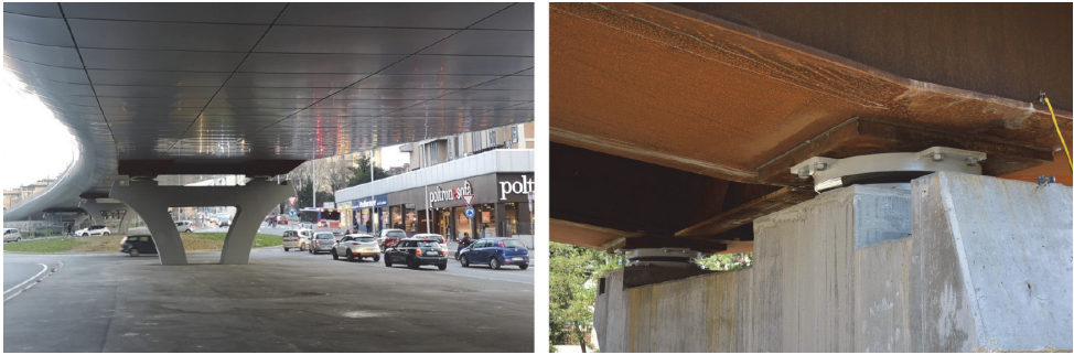
Figure 10. The Terzolle-Mugnone Viaduct, Italy (left), and detail of the pendulum isolators installed in it (right) (courtesy of Matildi+Partners, Italy)
