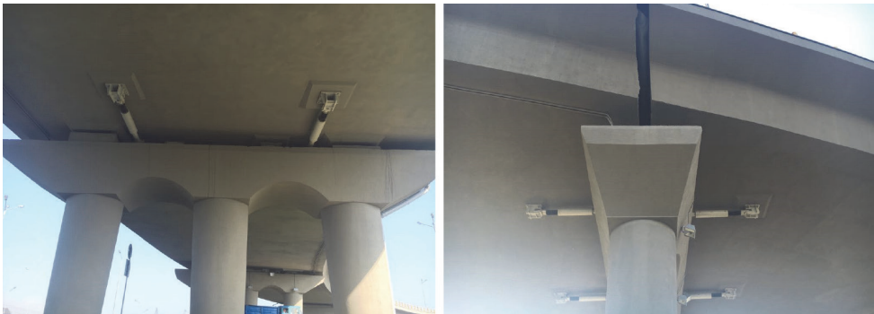
Figure 8. Viscous dampers and isolators as installed in the Saina-Ryskulova Bridge, Kazakhstan
