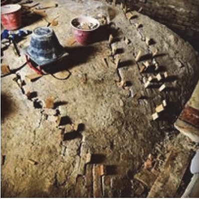
Figure 11. Rocca of Sissa Cracks in the extrados of O.G vault
