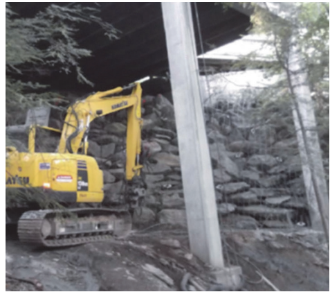
Figure 8. Slope stabilisation under a newly built residential car park. No damages were observed during and after the earthquake. The potential damage of slope failure would have resulted in the collapse of the residential compound and the car park
