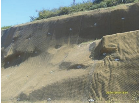
Figure 10. Previously installed Tecco system, which did not sustain any damage during and after the earthquake. The slope remained stable
