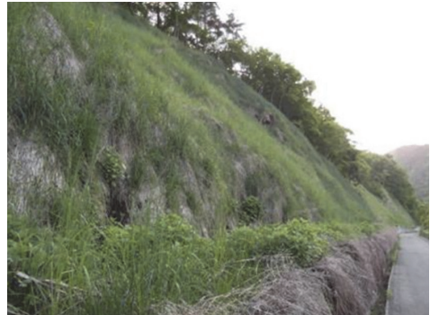
Figure 5. Not far away, a stretch of road where the slope stabilisation was done with high tensile steel flexible system and soil nailing and has long been revegetated, in Tono City. The whole stretch of slope along the road remained stable throughout the earthquake swarm
