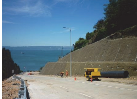
Figure 11. Overview of the stabilised road stretch. No deformation or failure after the earthquake
