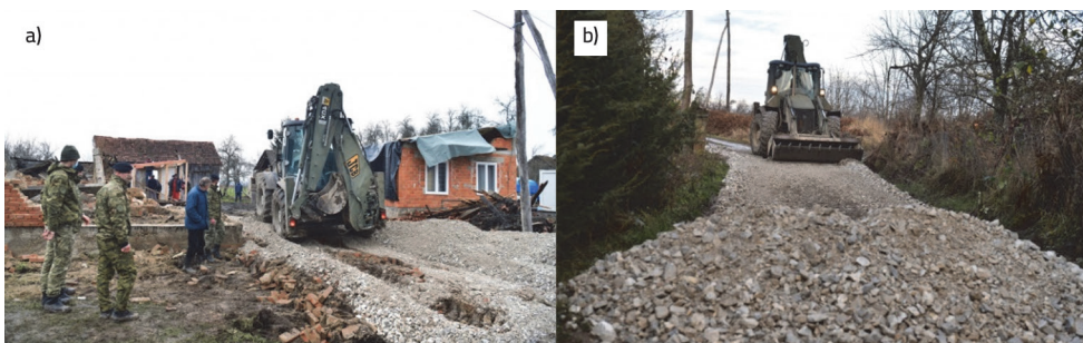
Figure 3. Reconstruction of the roadways mechanically – with machines; a) in settlements; b) out of the settlements
