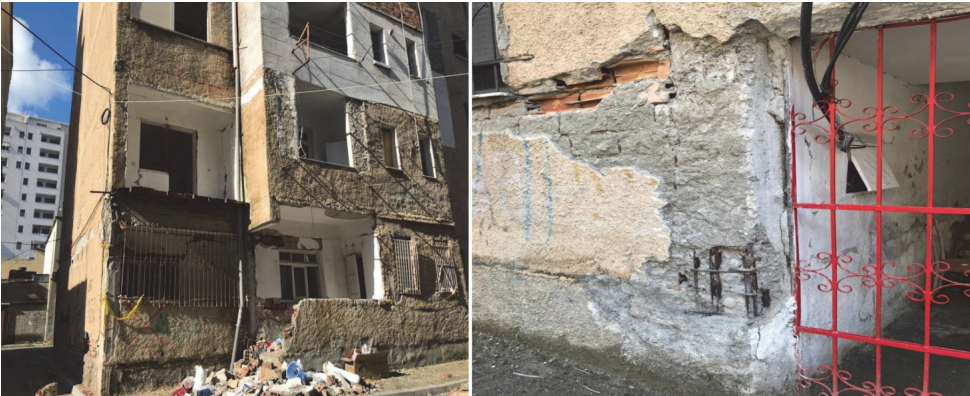
Figure 7. Damages in a masonry structure
