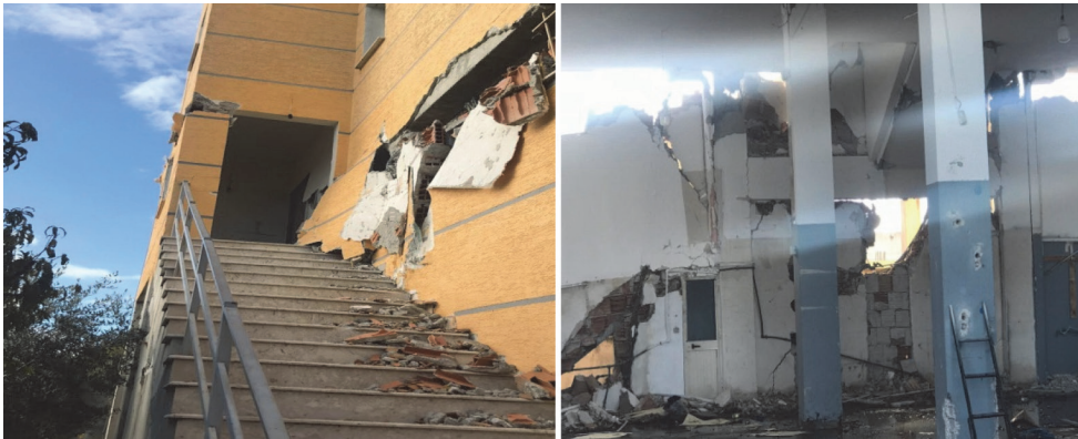
Figure 5. Damages occurred in a RC frame structure
