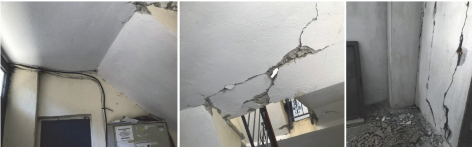
Figure 2. Damages in stairs and columns
