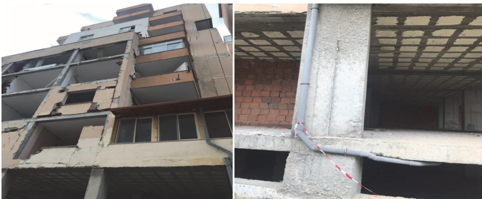
Figure 6. Damages in a RC frame structure with central core
