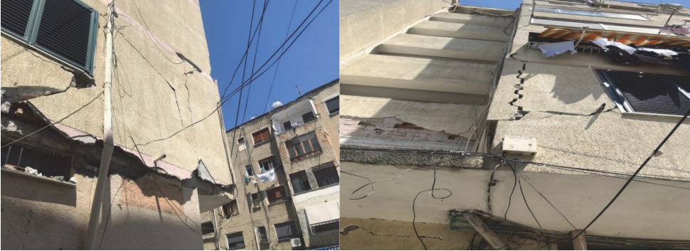
Figure 1. Exterior damages on 6 story building with combined structure
