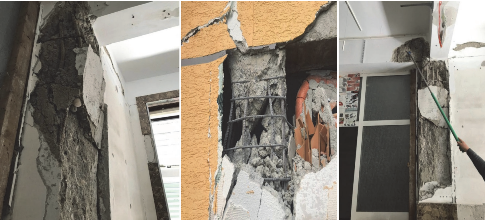
Figure 4. Damages in columns in RC frame structures
