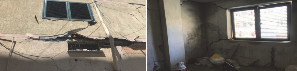
Figure 3. Damages in masonry exterior walls
