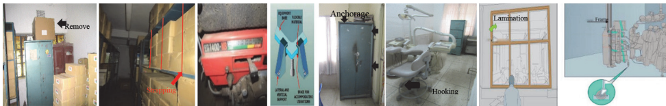
Figure 5. Mitigation technique for Removal, Relocation, Restricted Mobility, Anchorage, Hooking, Modification and Safety of Operation Theatres, Source. Field Survey, 2019 and [4]
