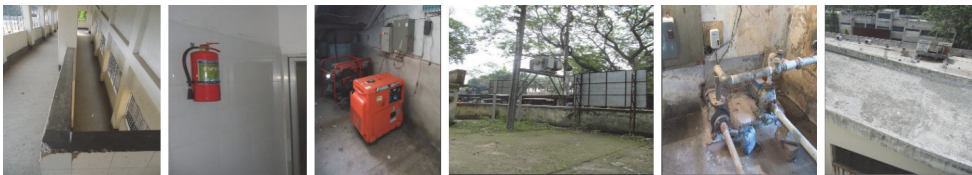
Figure 1. Ramp of the exit system, Fire fighting system, Generators and Transformer and Water Supply (Source. Field Survey, 2019)
