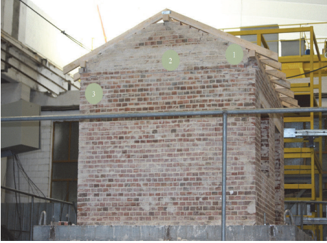
Figure 8. South wall with inclined cracks highlighted
