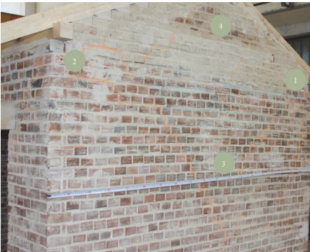
Figure 9. North wall with inclined cracks highlighted
