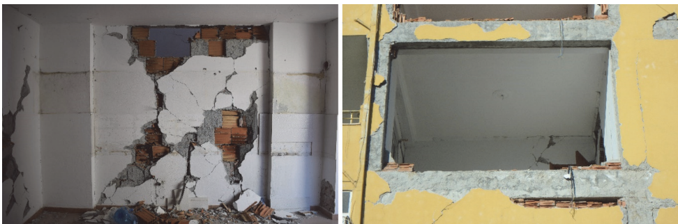
Figure 2. Observed very heavy damage or destruction of masonry infill walls
