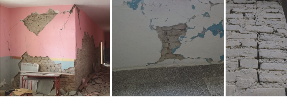
Figure 7. URM structures: a.) Heavily damaged URM [9]. b.) Pier cracks. c.) Corner failure
