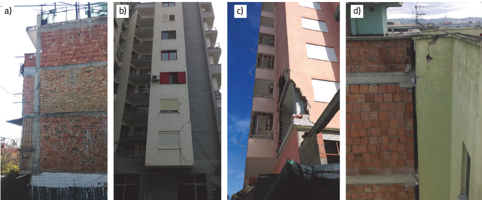
Figure 8. a.) Incremental construction. b.,c.) Damage in lower storeys. d.) Insufficient gaps
