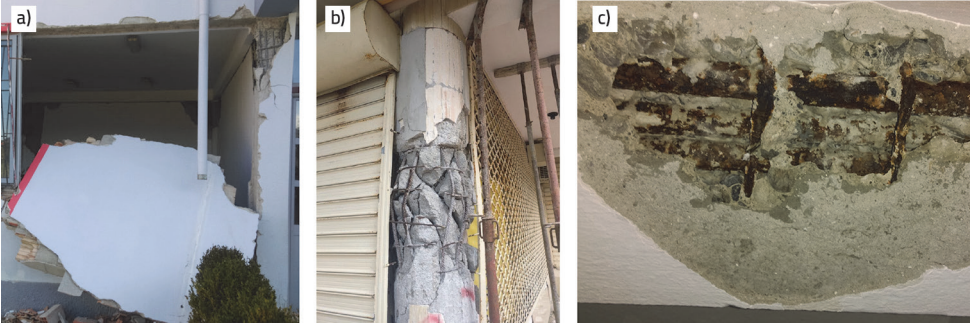
Figure 9. a.,b.) Buckling of reinforcement. c.) Corrosion of steel reinforcement.
