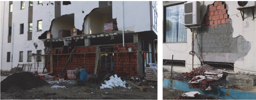
Figure 10. Non efficient attempts for damage remediation.
