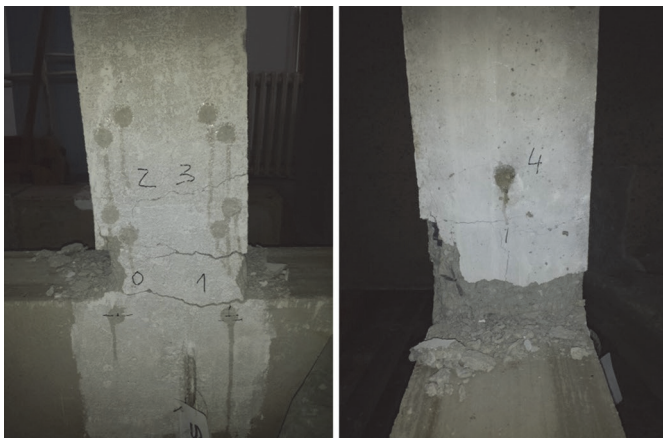
Figure 2. Localization of cracks in the plastic hinge zone of S3-A beam (front and side view)
