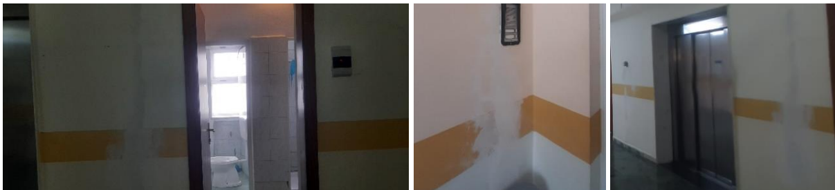
Figure 2. Cracks in the wall from the earthquake in 2019 Tirana, Albania.
