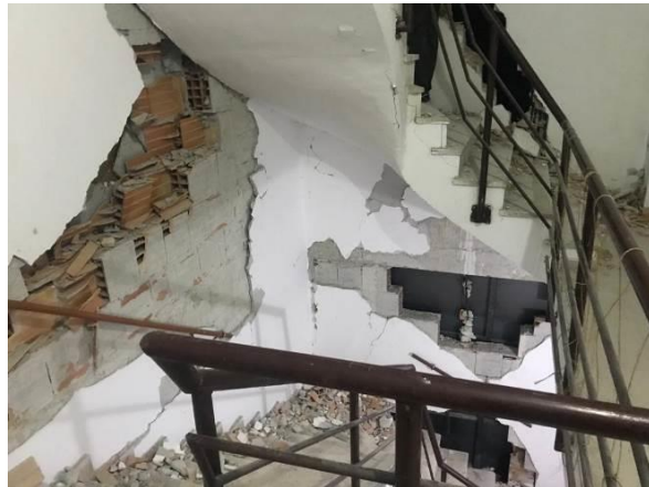
Figure 16. Inerts fallen down stairs.
