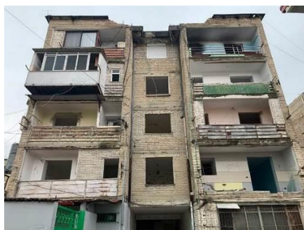
Figure 11. Collapsed brick parapet. 1970s construction building
