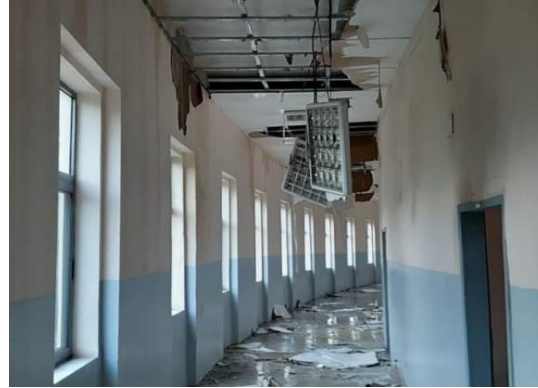
Figure 21. Collapse of suspended ceiling and light fixtures during the earthquake of September 21th, 2019. Faculty of Geology and Mining. PUT. Tirana. Source: http://redaktori.net/?p=17147
