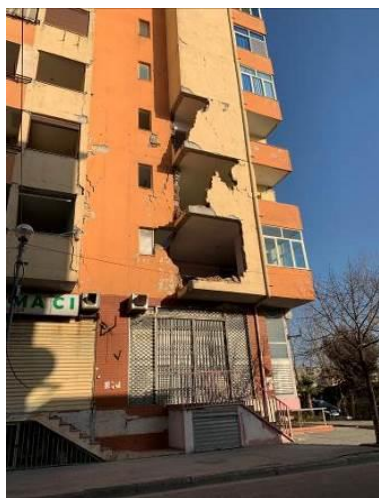
Figure 6. Walls collapse in the cantilever volumes
