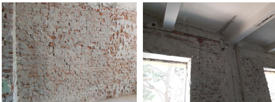
Figure 3. Cracks in masonry walls
