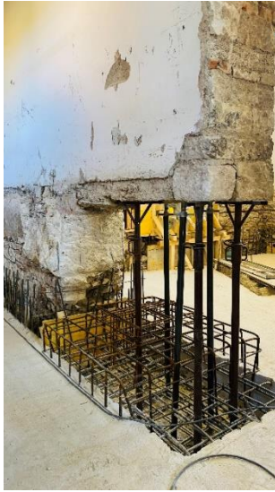
a) Demolition of existing foundation, new foundation reinforcement and support of masonry wall with props
