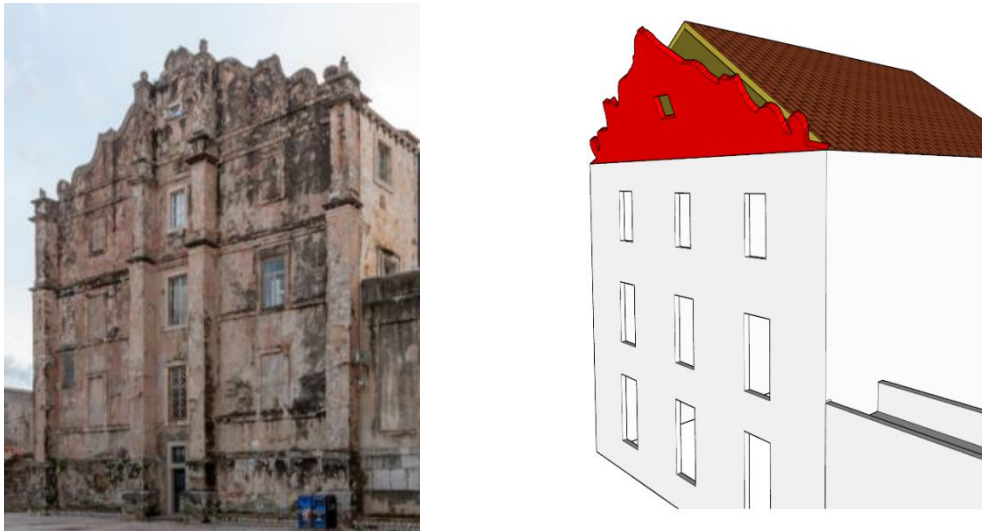
Figure 11. Description of the assumed local mechanisms LM1 and LM2. a) Clock wall; b) Gable Wall.
