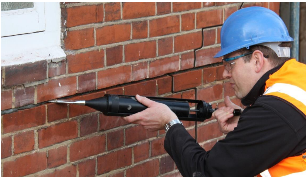
Figure 3. Thixotropic cementitious grout applied to a horizontal slot in preparation for insertion of helical bar.
