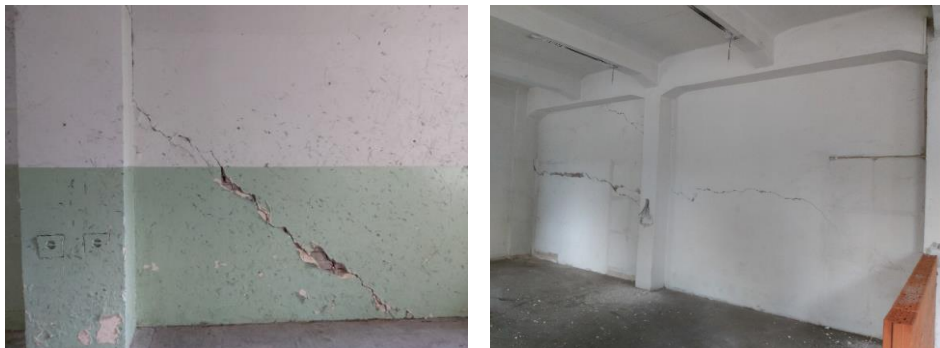
Figure 2. Horizontal and diagonal cracks
