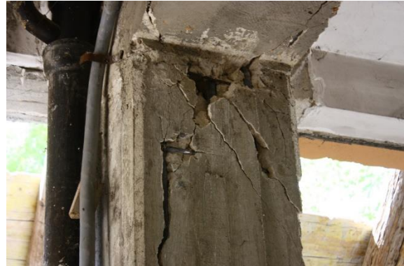
b) Brittle fracture in a pillar
