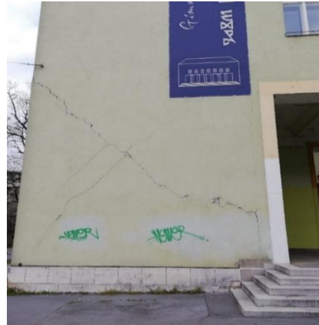
Figure 2. Typical damage on the load-bearing wall
