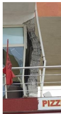
Figure 4. Damage due to "soft story" and torsional effect
