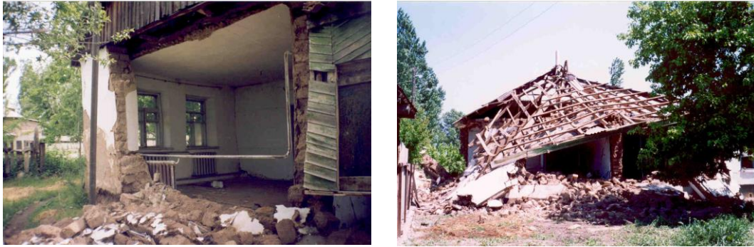
Fig. 4. Destruction of adobe houses as a result of the earthquake on May 23, 2003
