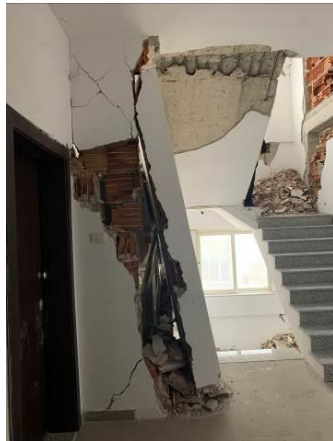
Figure 15. Damaged stair ramps
