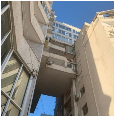
Figure 1. Collapse of the facade walls in the "connecting bridge" area
