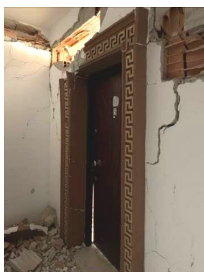
Figure 17. Exterior door with damaged lock
