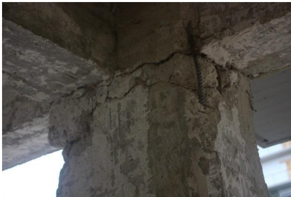
Figure 9. a) Brittle fracture in the top of a pillar
