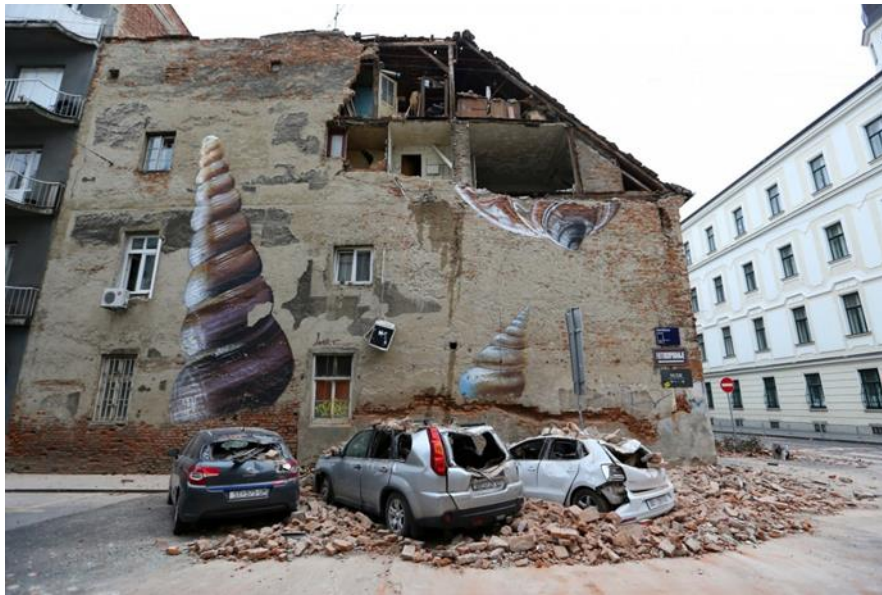
Figure 1. Masonry façade damage – Zagreb 2020 (Photo credit REUTERS/Antonio Bronic).
