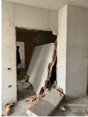
Figure 20. Collapse of the partition wall
