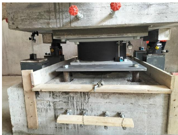
7) the isolator during installation: non-returnable flat jack has been already injected, while bottom anchorage grouting is not yet carried out.
