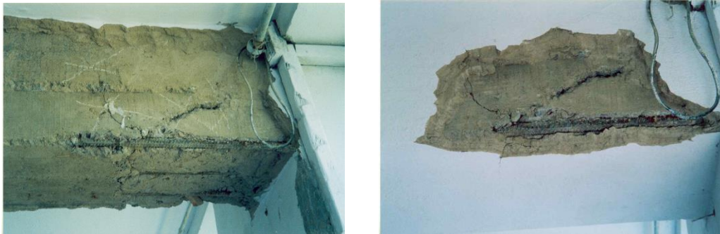
Fig. 9. Damage to the reinforced concrete crossbar in the School building
