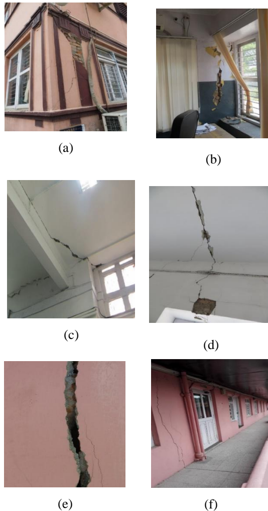
Figure 2. a) Heavy vertical crack in the pier; b) Vertical crack in the pier; c) Deep crack in the first floor slab;d) Crack in the slab; e) Crack width of about 20 mm in the wall; f)Vertical crack in the Wall
