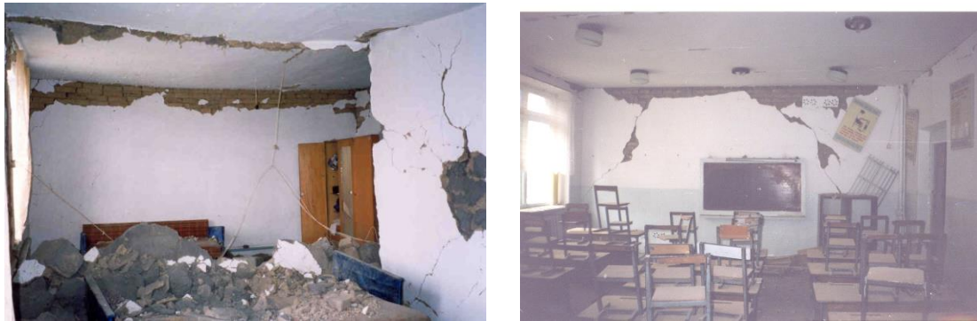
Fig. 8. Damage to schools with load-bearing brick walls.
