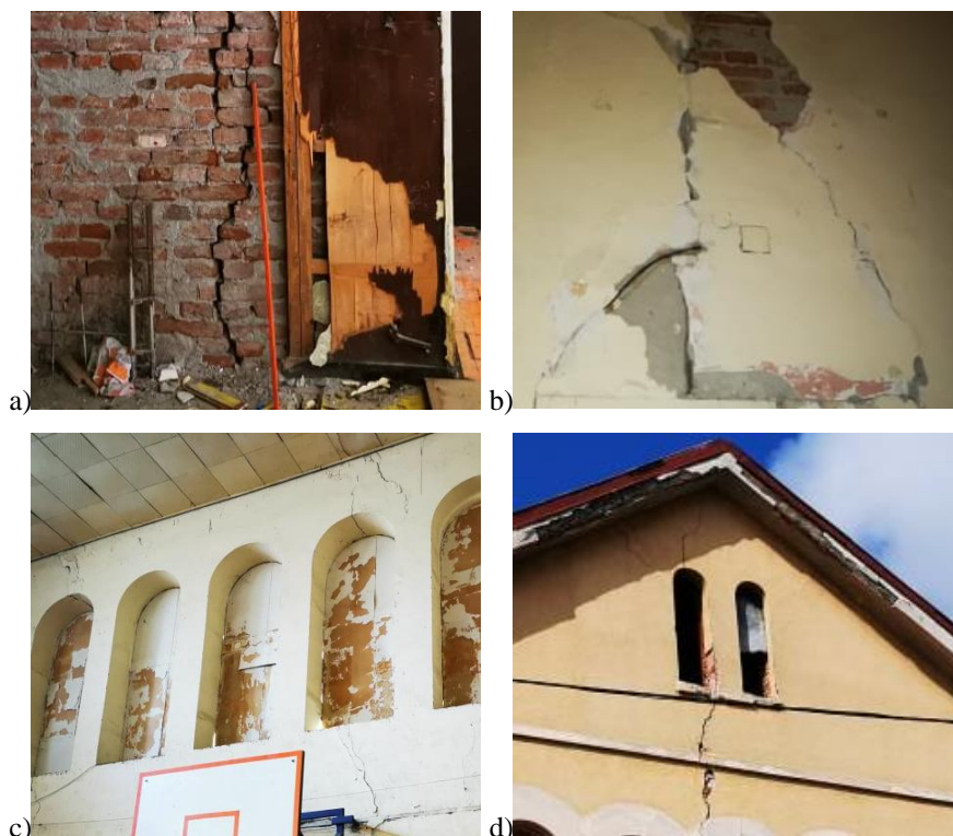
Figure 4. a), b), c), d) Severe cracks on the load-bearing wall elements
