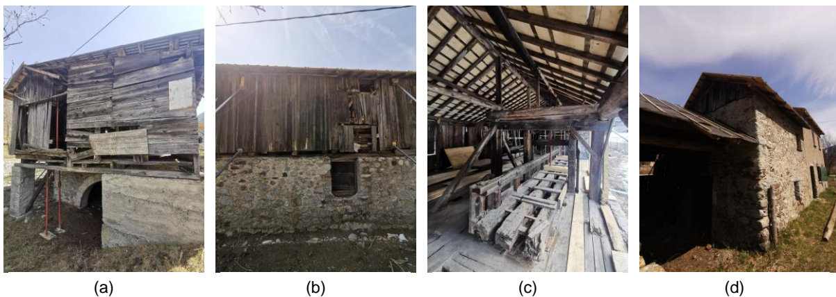
Figure 5. Front (a), side (b), and interior (c) views of portion A of the sawmill; view of portion B (d).
