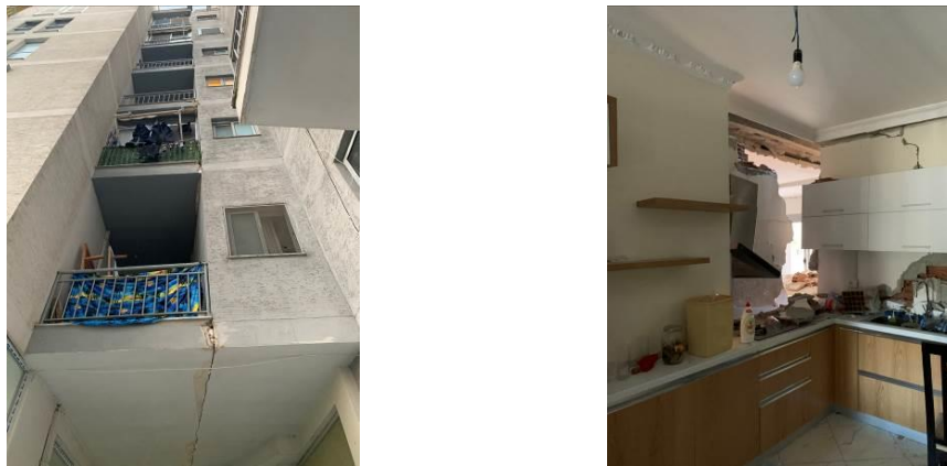
Figure 8. Damage caused during the collision in the joint position
