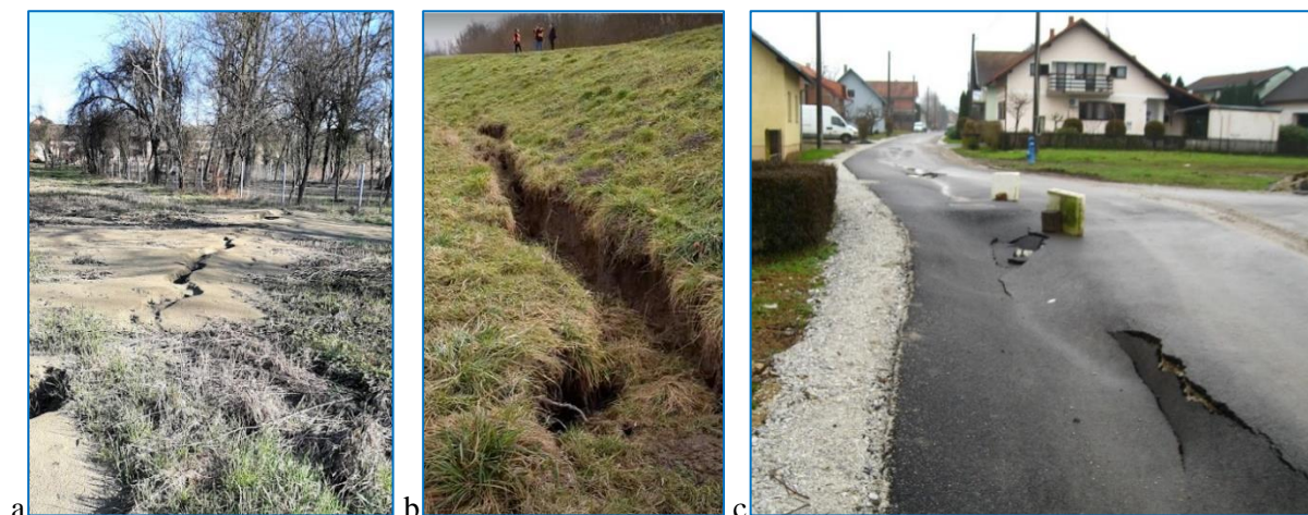
Figure 1. Examples of liquefaction in Petrinja earthquake: a) ejecta in the field in Hrastelnica, b) cracks in the levee in Sisak along the Sava river (Galdovo), c) subsidence of the road in Petrinja (Drenčinina)
