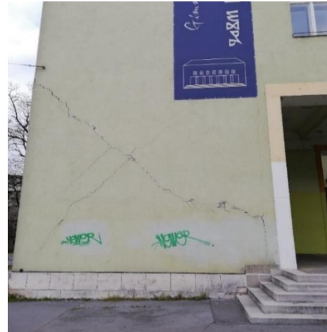
Figure 2. Typical damage on the load-bearing wall
