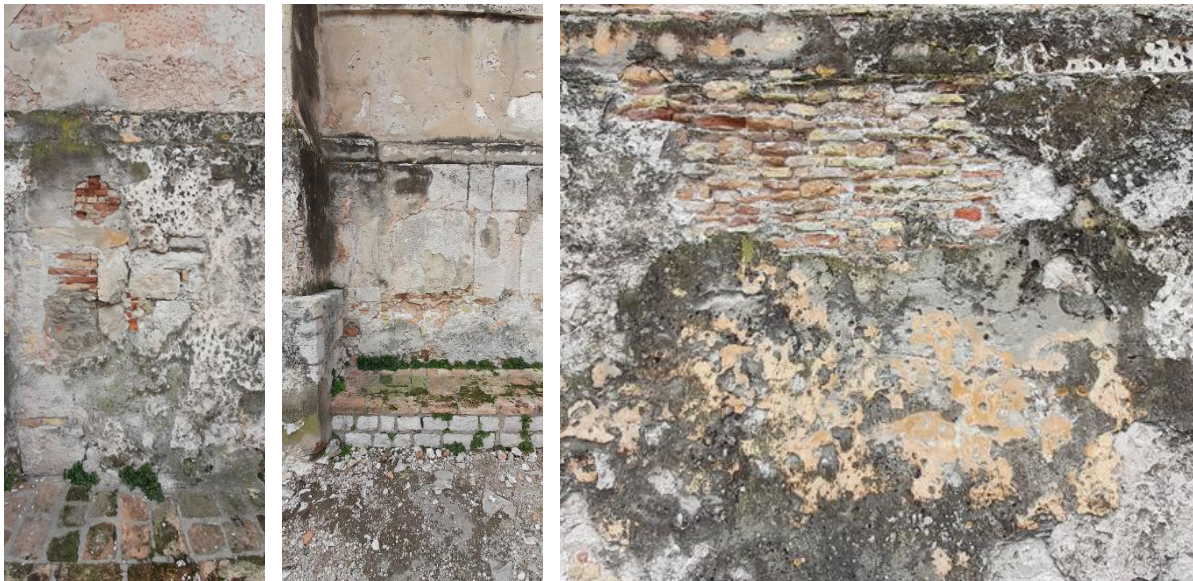
Figure 2. Materials characteristics of the external walls (composite clay bricks and stone masonry of variable sizes).
