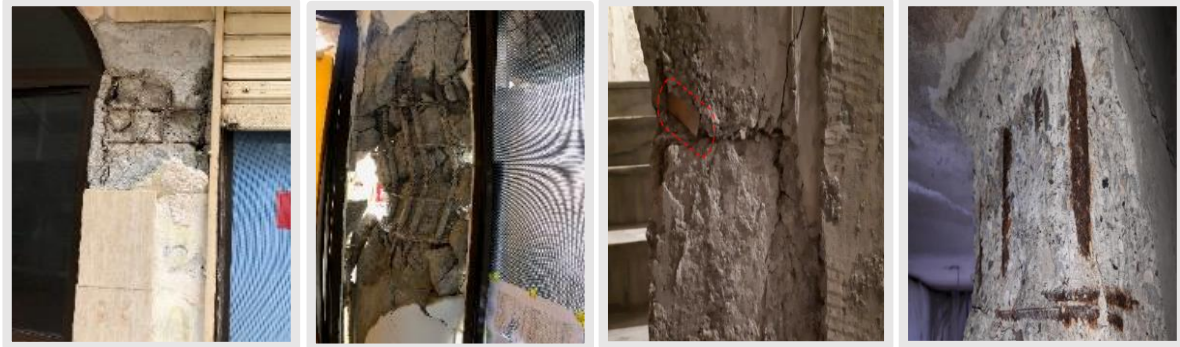
Fig. 5. Plastic hinge at the columns of multi stories building, inadequate materials and other deficiencies.
