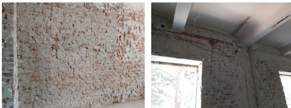
Figure 3. Cracks in masonry walls
