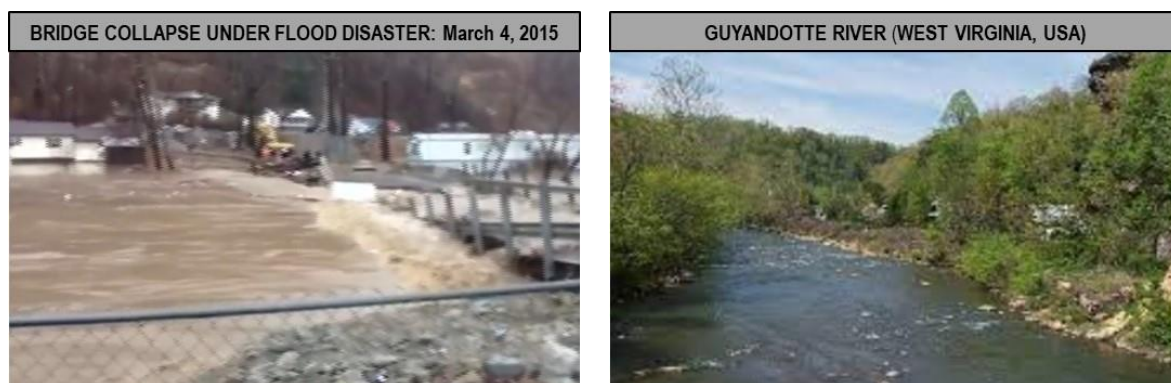
Figure 11. Typical loading of bridges under flood disasters: Collapse of the Guyandotte river bridge under flood, March 4, 2015 (left) and common water level of Guyandotte river in West Virginia, USA (right).
