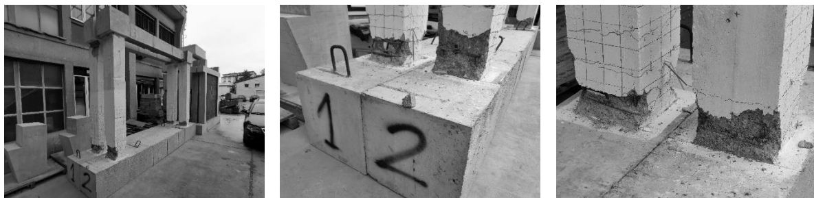
Figure 8. Crack propagation and damage in frames
