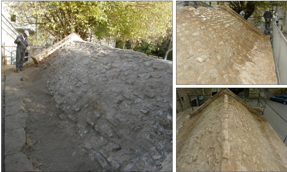
Figure 4. Extrados of the vault during the replacement of the roof tiles in 2008 [6].
