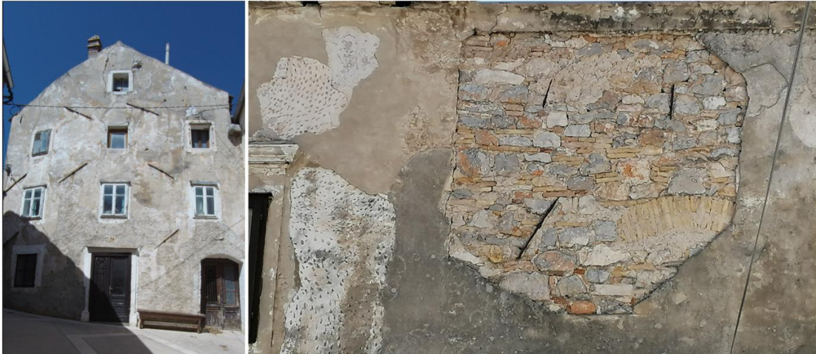
Figure 6. Tie rods visible on the facade of the building (left) and inside the section of the Wall (right)
